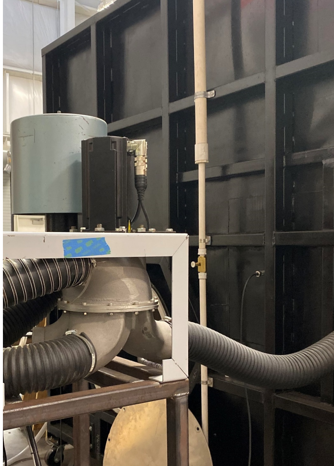
Pressure Valve with Connection to Pressure Box
